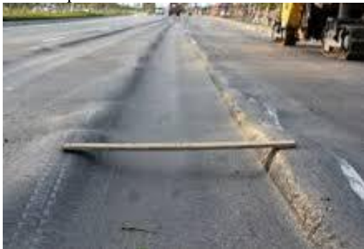
Fig.1. Rutting in flexible pavements
