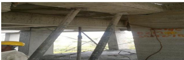
Fig. 2.6.1 Problem arises if supports are not provided to the beam prior to placing of staircase.
